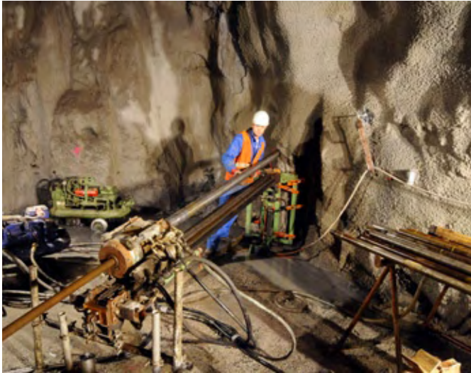
Geotechnical investigations for Unit 11, drilling work in the new exploration gallery (March 2008).
