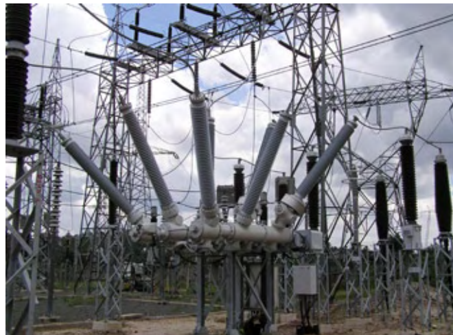
High Voltage connection with 220 kV hybrid gas-insulated switchgear.
