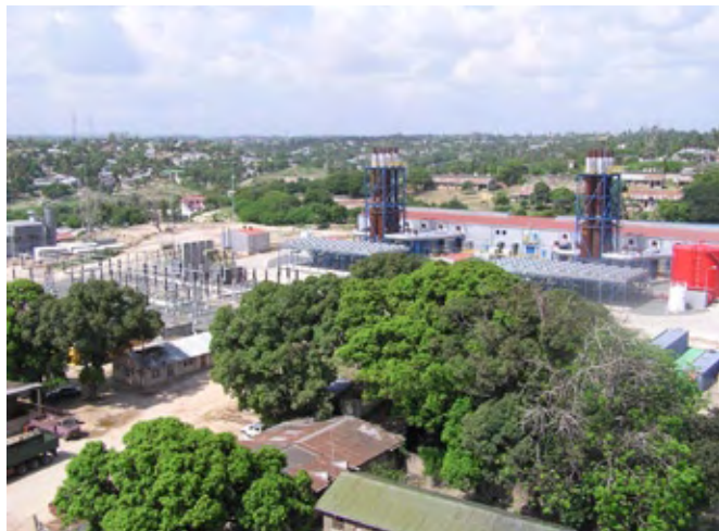
Ubungo 100 MW Gas Engine Power Plant.
