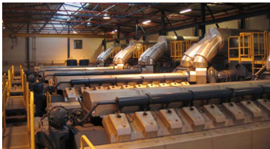
Gas Engine Hall.
