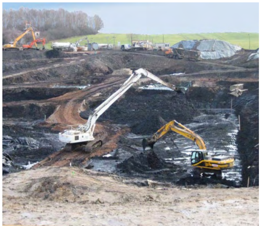
After the extraction of tar products the backfilling of the dumpsite is prepared.
