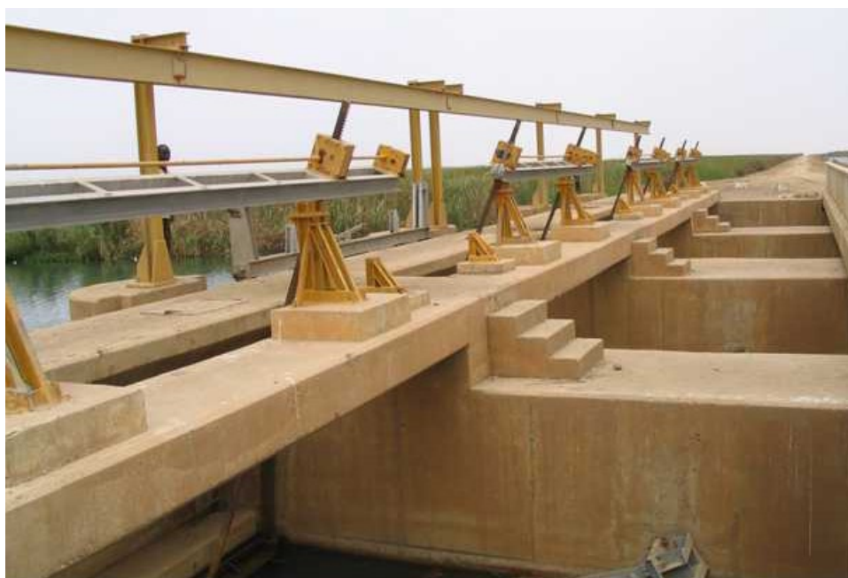
Raw Water Intake on River Senegal.
