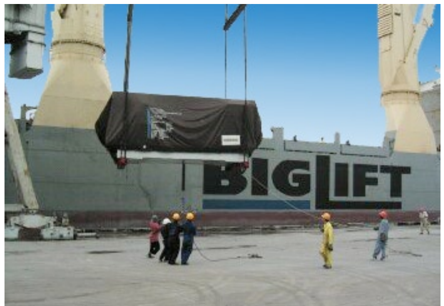
Arrival of the first gas turbine in Calabar.
