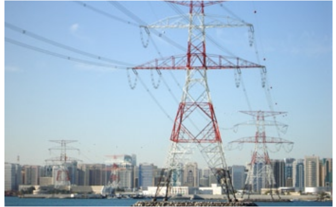
Parts of the 400-kV transmission line network of Abu Dhabi city.
