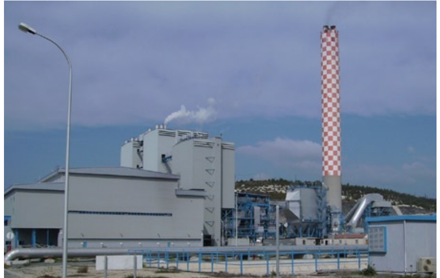
Vasilikos Power Station, Cyprus. Within the next 10 years it is envisaged to install three combined-cycle power plant units, each with a capacity of 200 MW.
