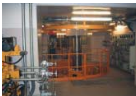
Interior view, powerhouse
