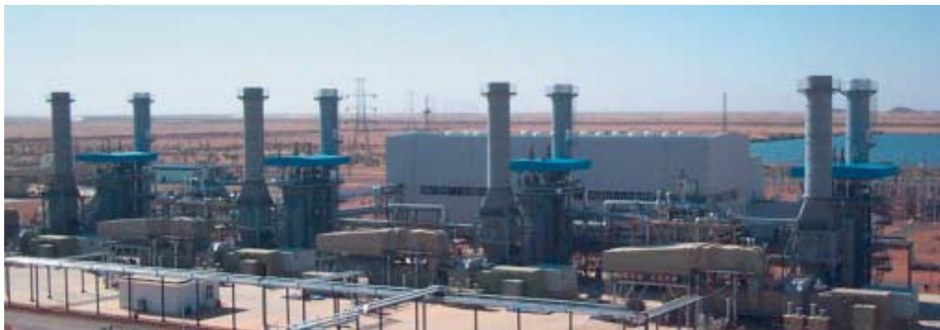
The existing 190 MW CHP station Garri 1
