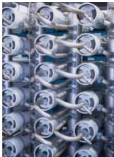
Stack of pressure vessels
